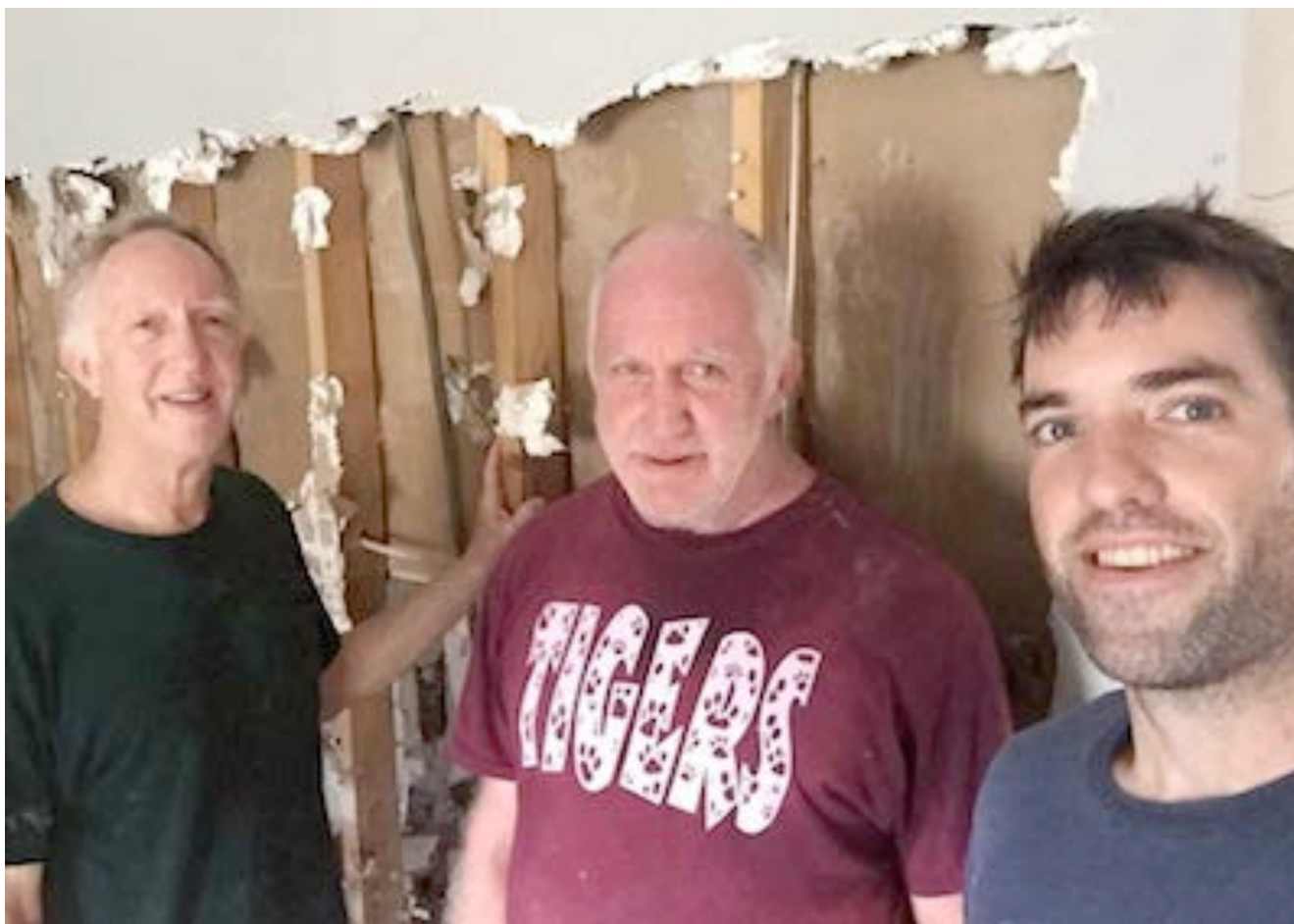
Everyone and anyone in the Baton Rouge area was ripping out sheet rock after the water receded. Here are Times business manager and photographer Mike Dooley (L), his brother Pat (C), and son Jake, Times cartoonist, doing some demolition and male-bonding.
